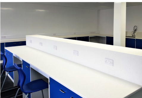
Velstone worktop - raised divider/power outlets
