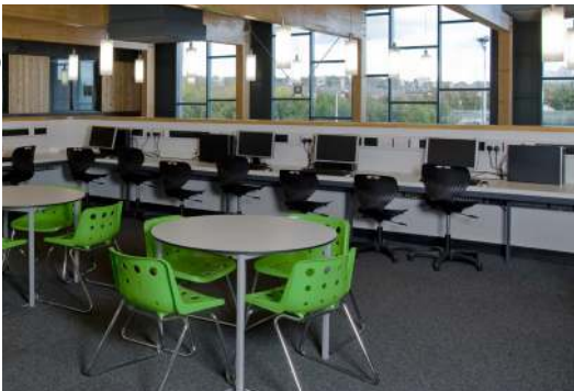
Wall mounted trunking
