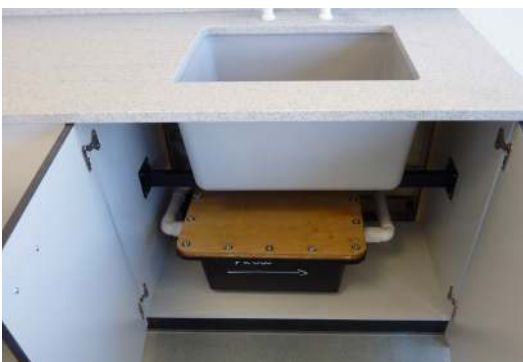
Large sink with clay trap
